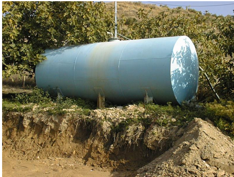
Figure 8: Storage Tank at Judayta pumping station
