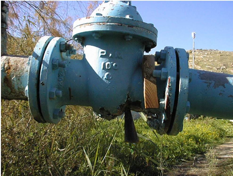
Figure 12: Water Meter at Well No. 1
